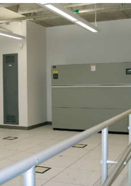
This room in Coover Hall will house the High-Performance Computing Center.
