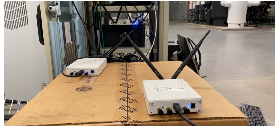
Fig. 5: PV-RAN testbed at ISU Research Park
